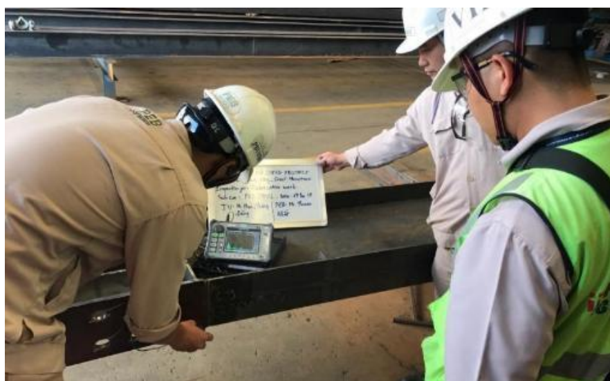
06-C Welding Inspection – Ultrasonic Test Ultrasound used to detect internal flaws in welds for quality assurance
