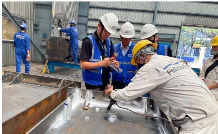
06-B Welding Inspection – MT Test Magnetic Particle Testing to detect surface/subsurface defects
