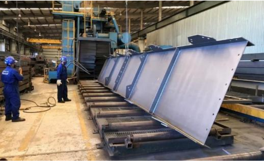
08-A Shot Blasting (Normal) Rust and scale removal before coating Maximum web width: up to 1800 mm Maximum flange width: up to 2500 mm
