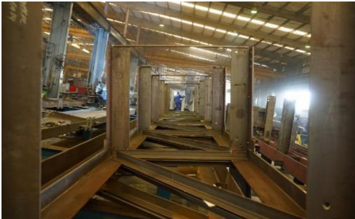
04 Fit-Up Process Aligning components before final welding Critical for beam straightness and structural integrity
